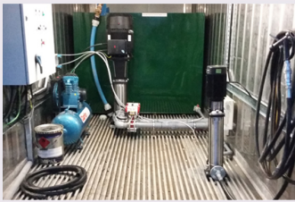
Secure Pump House
